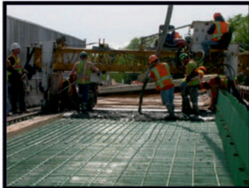
Figure 4: Internally Cured Concrete being Cast at Bartell Road in New York (Wolfe, 2010)
